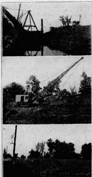
FIG 1. (Above) Constructing a levee with a dredge boat. (Center) Repairing a levee with a caterpillar shovel. (Below) A new levee.
