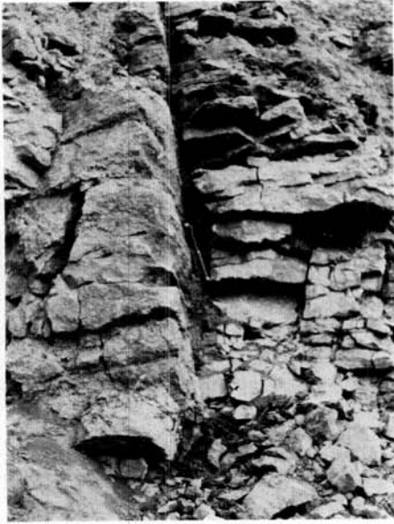
FIG. 5.—Filled joint at Site 2. Pick at contact of gray-brown pebbly clay above and reddish-brown silty clay below.
